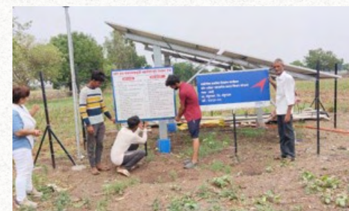
Solar Powered Irrigation site under Project Saakshyam
